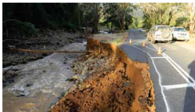
Flood damage on Murphys Creek Road
